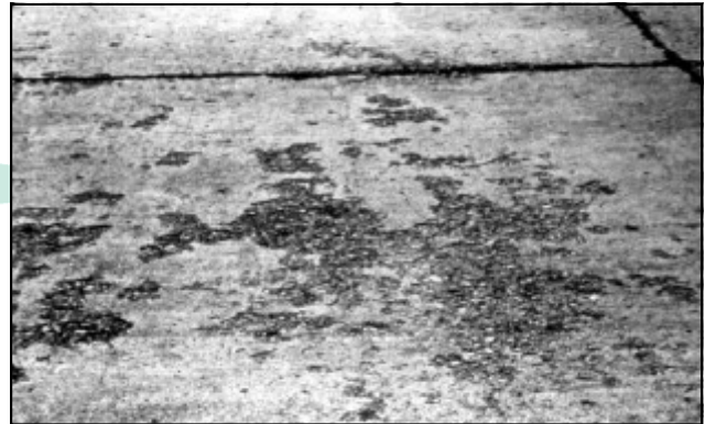
Scaling on Concrete Slab
