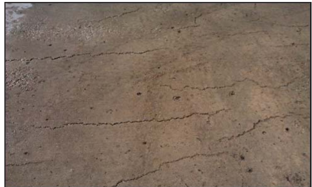
Plastic Shrinkage Cracks
