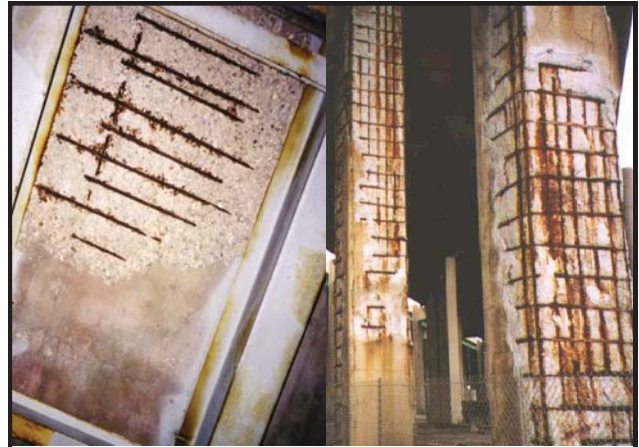
Reinforcement Corrosion in Structures
